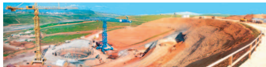
Station de pompage Beni Haroun, Algérie
