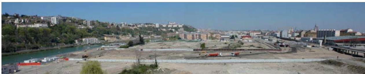
View of the site before excavation to create the basin: grid of soil quantities to be excavated using suitable authorised channels, leakproof storage areas, riddling, monitoring of the excavated soil, monitoring of water quality during the whole works period.
